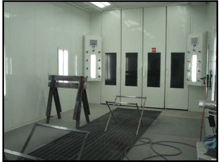
Inside view of one of the paint booths
